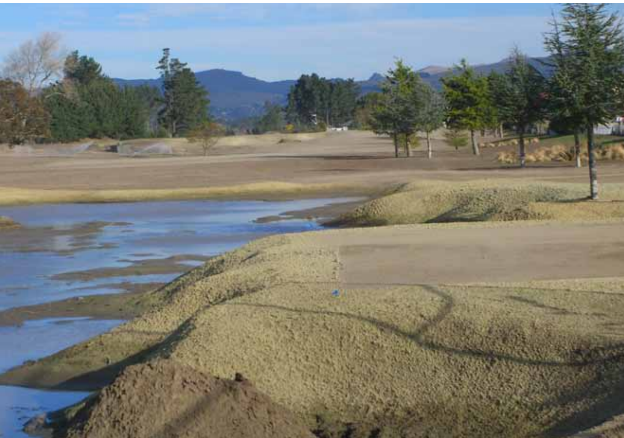
Above: it was imperative to 'raise' the profile of many of the holes at Waimairi after the earthquake. Construction works saw the 15th tee raised and also a wetland carved out.
